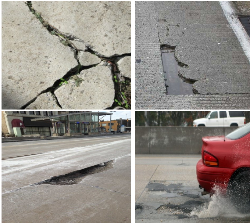
Figure 15 Water Related Damages; Potholes, Corner Breaking and Wide Cracks.
