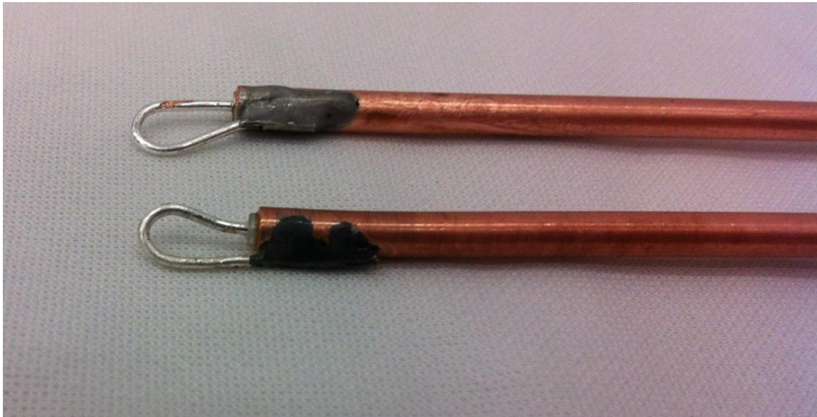
Figure 40: The Loop Couplers Used in the Second Cold Test. The Probe Coupler (Top) Remained the Way It was Installed, the Input Probe (Bottom) Was Discolored Significantly
