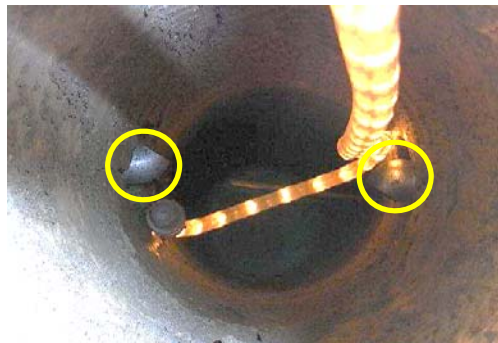
Figure 23 – Two pieces of 1/4" 90-degree galvanized installed inside the combustion chamber (adapted from Barth, 2009)
