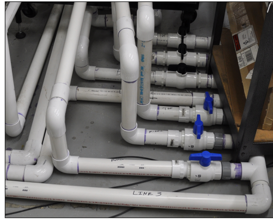
(b) PVC valve arrangement showing valve controls for 2 of 3 lines. Each line has three valves, allowing gas to be injected into any sub-stream. The configuration shown is allowing gas from lines 3 and 1 to enter the bottom sub-stream.
