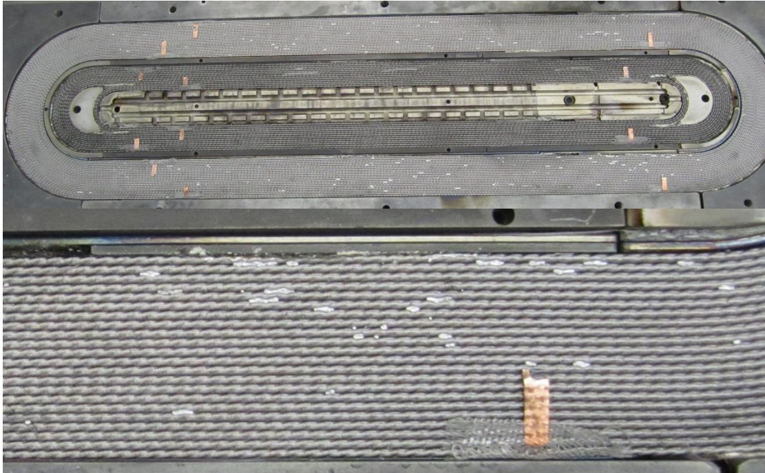
Figure 85: Leaked Tin in the Body of the Outer Coil in TAMU3c
