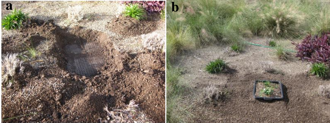
Figure 3.1 Installation of planting containers. Media was excavated down to the filter fabric layer (a). Planted containers with uniform media were placed directly on top of the filter fabric layer (b)
