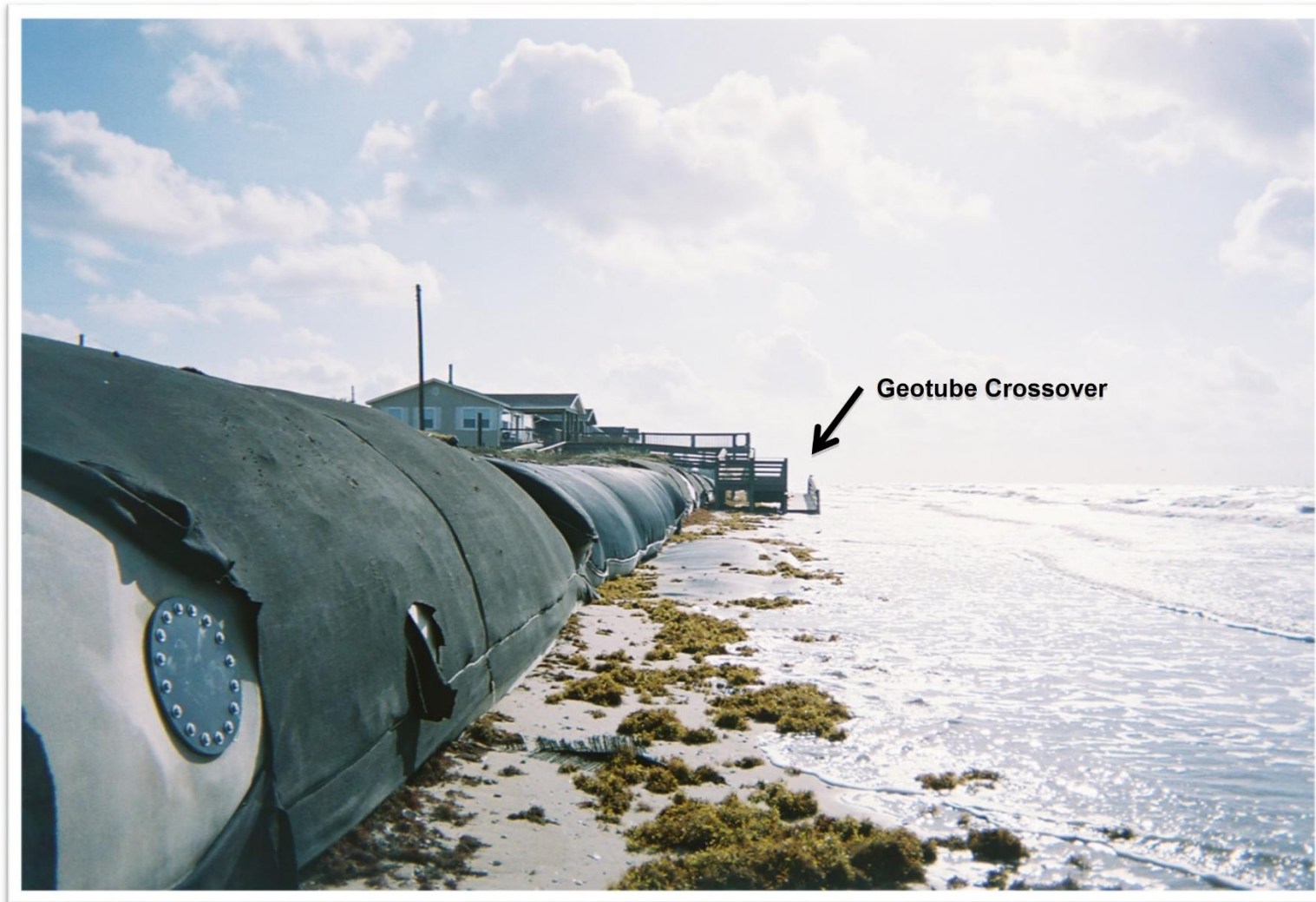
Figure 3.10. Geotextile tube and associated crossover (in background) on Bolivar Peninsula section B28 (poor quality) under high tide conditions 9 June 2008. (Photo by Christi Hughes.)
