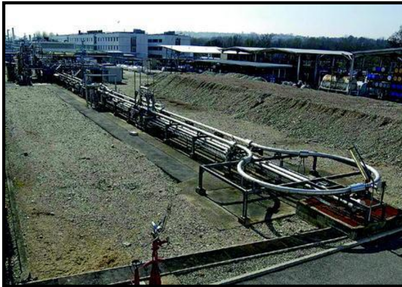
Figure 20: Real plant large scale multiphase flow loop, France [10].
