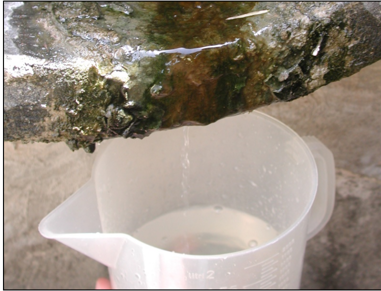
Figure 12. Valve leak measured from test 16HC1 (Leigh and Fipps 2008a).
