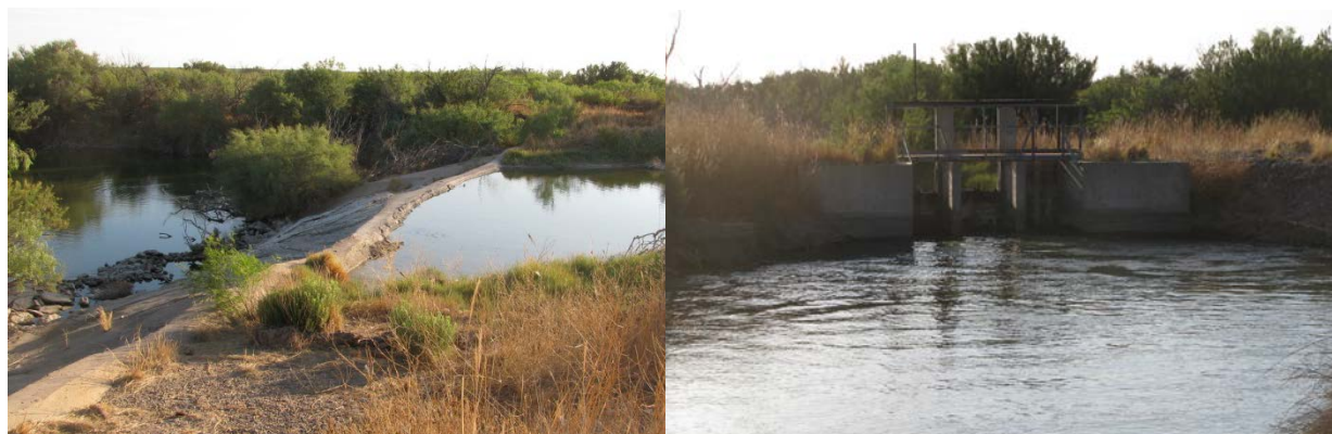
Ward II Irrigation Turn Out just upstream of the FM 1776 road crossing
