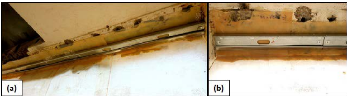
Figure 7.54. FS15. (a) Mechanical anchor at top support. (b) Close-up of deformed anchor.
