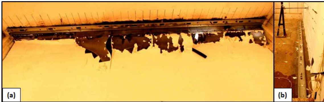
Figure 7.38. FS11. (a) Five of the seven sheets of film peeled off the top of the CMU wall. (b) Film at the bottom support did not appear to peel back.
