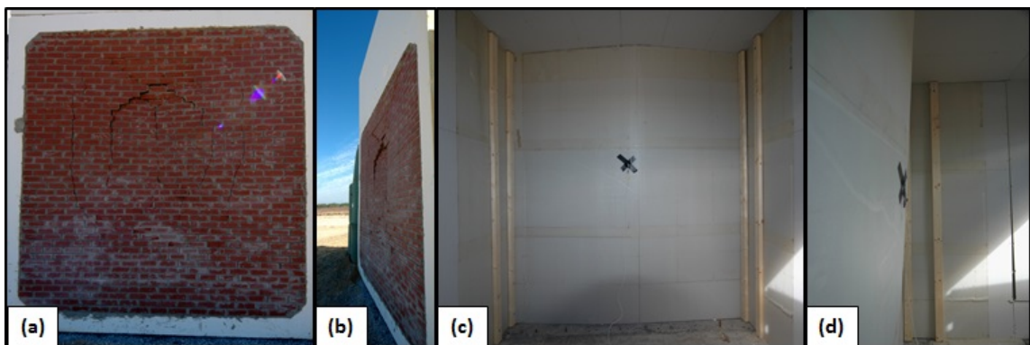
Figure 9.8. Retrofitting wall response. (a) Posttest exterior of retrofitted wall. (b) Profile view of wall. (c) Posttest interior view of wall. (d) Retrofitted wall deflected into structure, but no debris fragments were found inside protected space.
