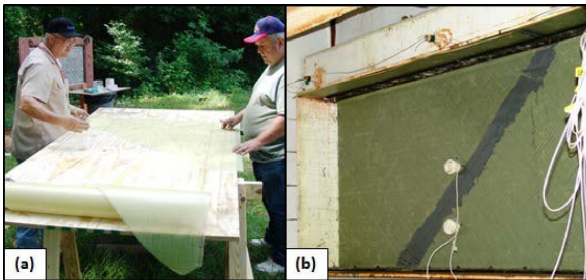
Figure 6.38. DW14. (a) Cutting film to orient fibers 45 deg to the horizontal mortar joints of the wall. (b) Two sheets of film used to cover CMU wall with epoxy seam along the center.
