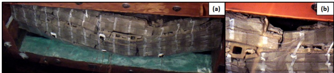
Figure 5.67. SW18. (a) Retrofit failure occurred when the film tore along the top support. (b) Tear in the elastomeric film.
