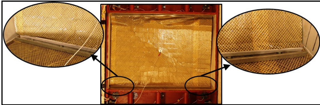
Figure 6.71. Interior view of retrofitted wall BLS8 and the damaged anchor plates.
