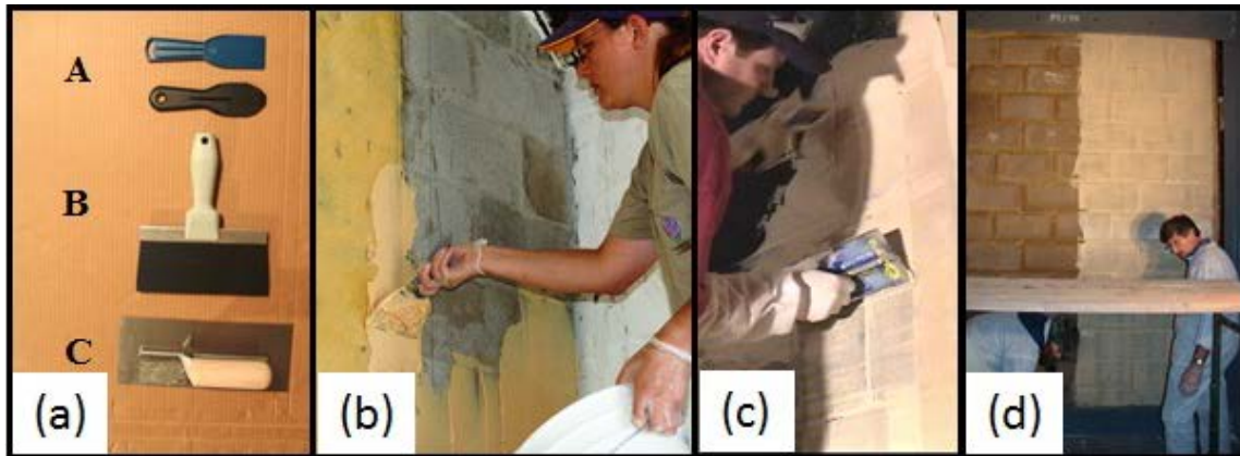
Figure 4.50. Trowel-on material application. (a) Trowels used to apply the thermoset. (b) Flat trowel used to apply material to wall. (c) Notched trowel used to control thickness. (d) One section of trowel-on material is completed and ready for film application.
