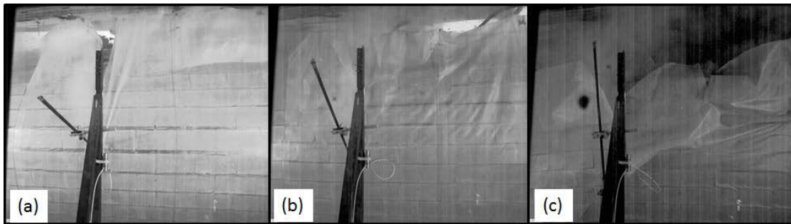
Figure 7.57. FS16: Frames from high-speed camera. (a) Blocks begin to disengage from the film. (b) Tear in film propagates the full length of the support. (c) Film and blocks fall into reaction structure.
