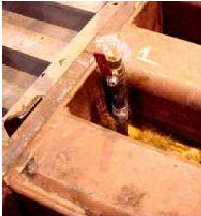
Figure C54. Close the relief valves when water begins to flow from relief valves.
