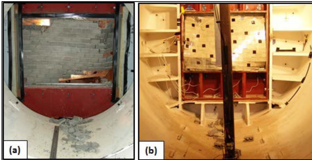
Figure 6.68. BLS7. (a) Damage to CMU wall. (b) Debris found in target vessel.
