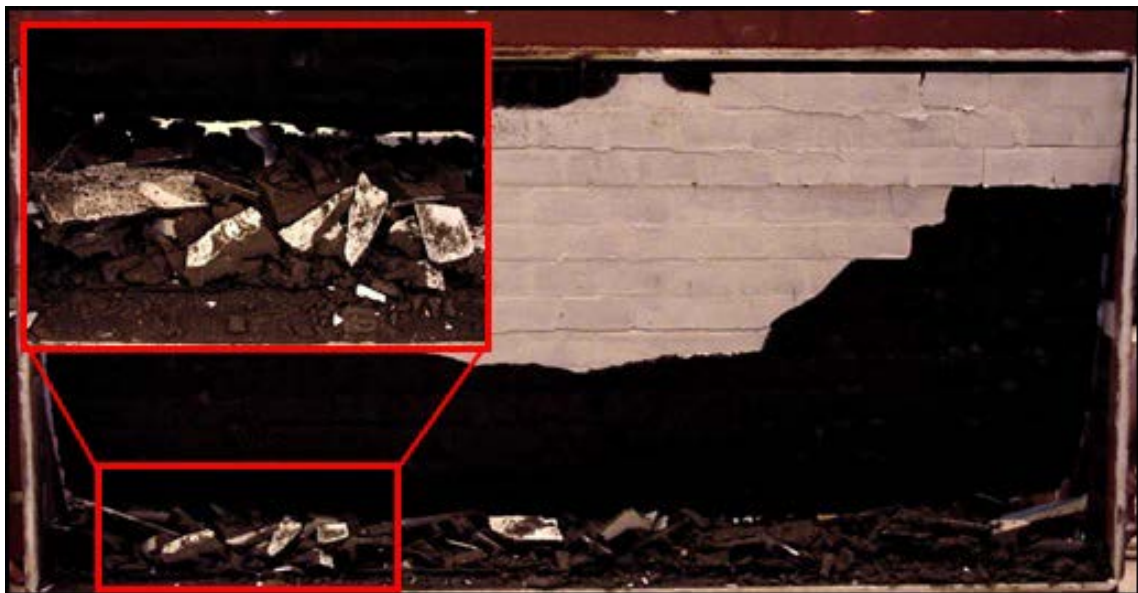
Figure 5.29. Accumulation of CMU debris on bottom flange of frame.
