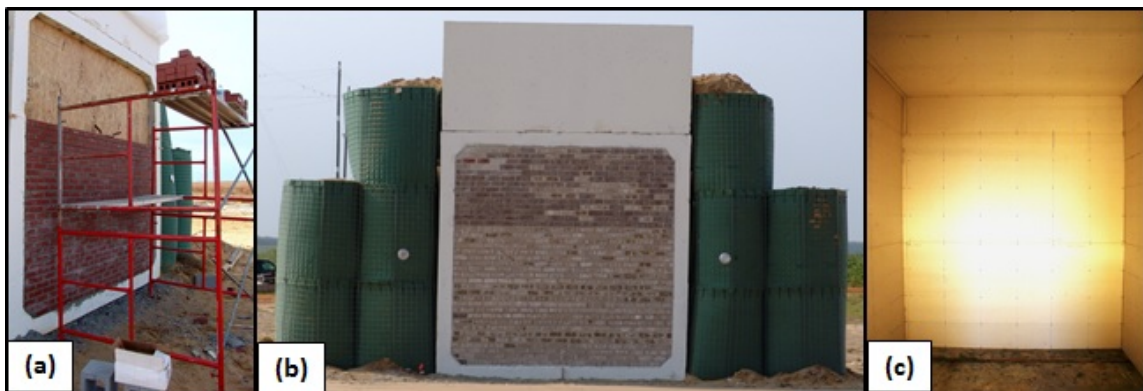
Figure 9.4. Brick façade. (a) Single wythe brick veneer. (b) Target exterior. (c) Target interior.
