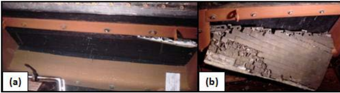
Figure 5.5. Trial 1. (a) Failure began at top support. (b) Complete failure of the retrofit material at the top support.
