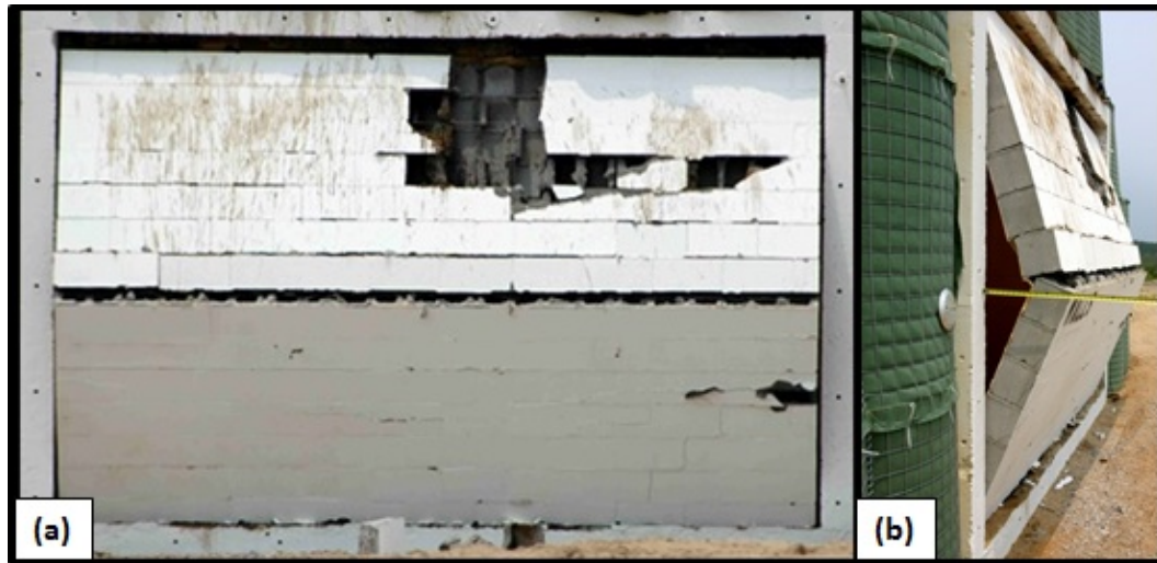
Figure 7.33. FS10. (a) Posttest exterior view. (b) View of permanent deformation.
