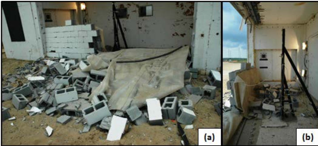
Figure 7.58. FS16. (a) Half of the wall fell out of the reaction structure. (b) Half of the wall fell into the reaction structure.
