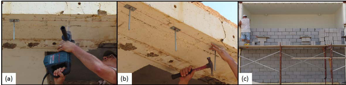
Figure 4.5. Full-scale construction. (a) Concrete hammer drill. (b) Installing anchor bolts to mount slip dowels. (c) CMU stacked in running bond.
