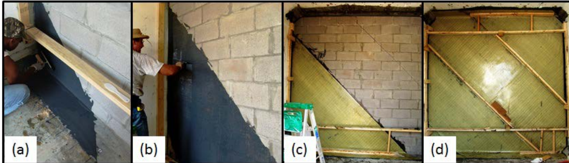
Figure 4.61. Retrofit application. (a) Trowel-on material applied in triangular sections. (b) Applying trowel-on material for film sheet two. (c) Sheet 2 applied to wall. (d) Temporary bracing applying pressure to film until epoxy cured.
