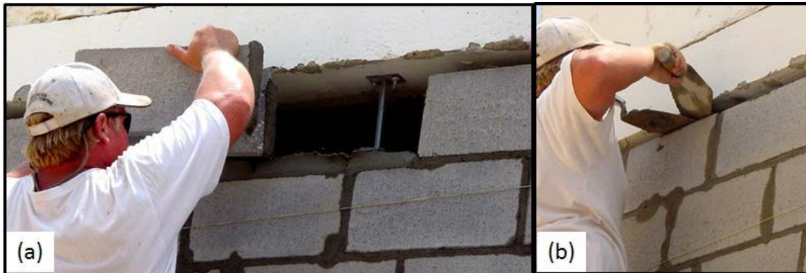
Figure 4.6. Wall construction. (a) Mason placing top course of blocks with slip dowels. (b) CMU cells with slip dowels fully grouted.
