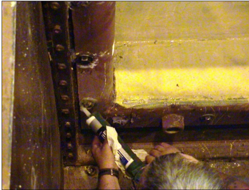
Figure C33. If a bolt appears to be stripped, then silicone bolts.
