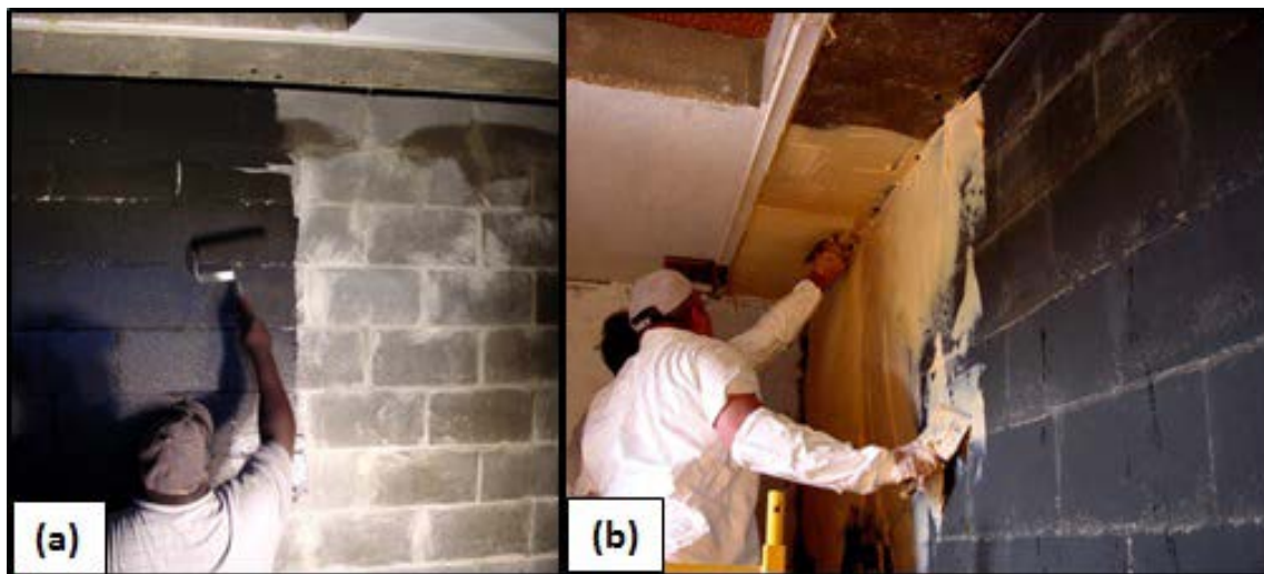
Figure 4.38. Quality control. (a) CMU wall surface is painted black; no paint applied to concrete supports. (b) Trowel-on material applied to the clean support and painted CMU wall.
