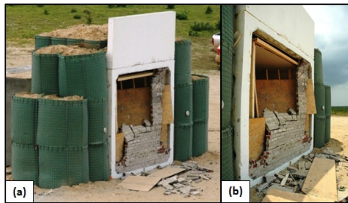
Figure 9.5. Unretrofitted wall response. (a) Posttest exterior view. (b) Debris outside of structure.
