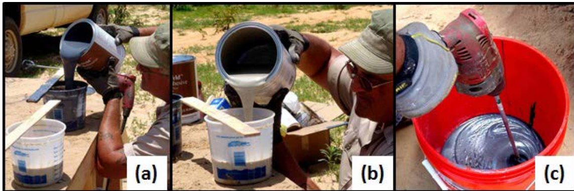
Figure 4.57. Mixing process. (a) Measure component A. (b) Measure component B. (c) Mix component A and B.
