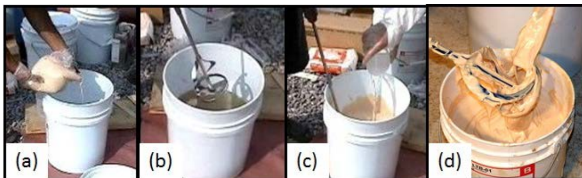
Figure 4.39. Mixing process. (a) Part B is added to Part A. (b) First two components are mixed with a paddle wheel attachment on the drill mixer. (c) Addition of Part C while mixing the material. (d) Material is ready to be applied to the wall.
