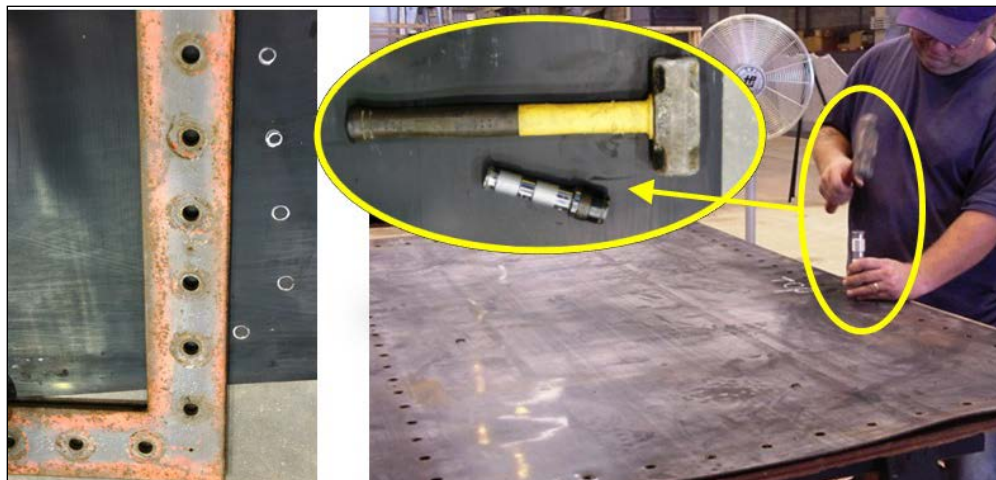
Figure C7. Use steel frame to layout bolt holes, then hammer and punch to create pass-through holes for bolts to secure the membrane to the HTC.
