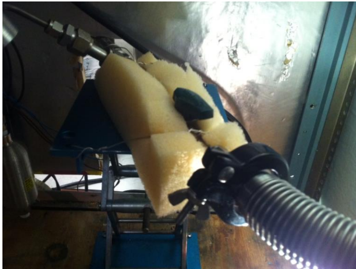
Figure D-10: Main Pump Valve Shown in the OPEN Position
