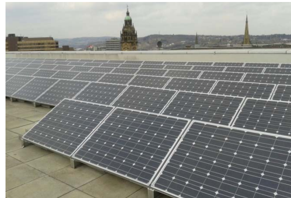
Figure 4 Case Study Building PV Array
