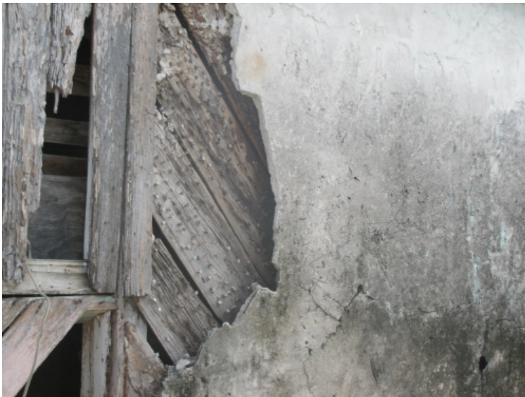
Fig. 6.14. Corner of the tailor shop at the Old Barry House showing the nails used to attach tar paper to the exterior walls, providing extra gripping surface for plaster.
