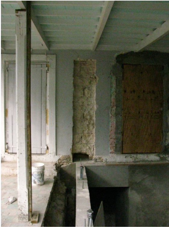
Fig. 6.13. Renovations at Java House reveal that the plastered exterior covers limestone blocks quarried from the cellar.
