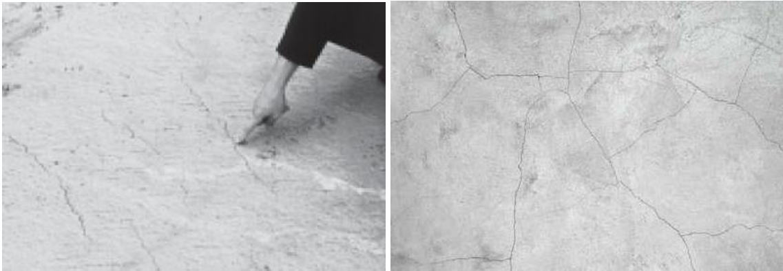
Figure 2-2 Typical forms of plastic shrinkage cracking
