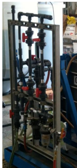
Figure 8. KASELCO piping system used to take sub-samples during treatment
