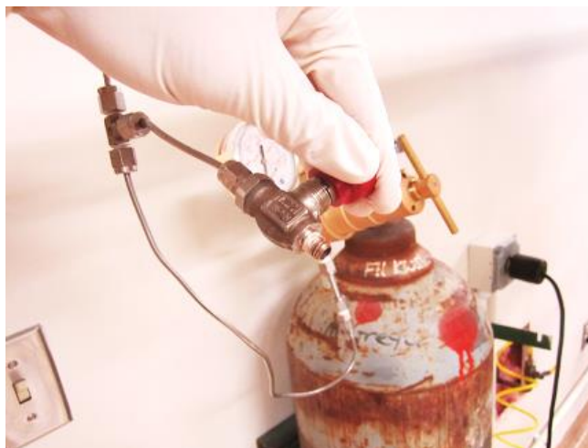
Figure 80: Open and Close Nitrogen Bleed Valve
