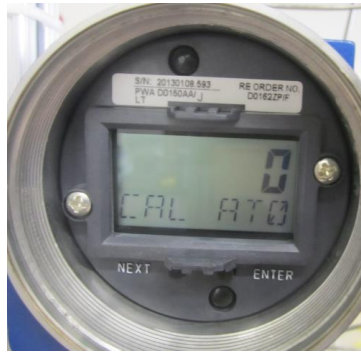
Figure 38: Pressure Transducer Panel
