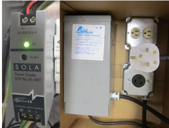
Figure 43: Power Supply and Transformer
