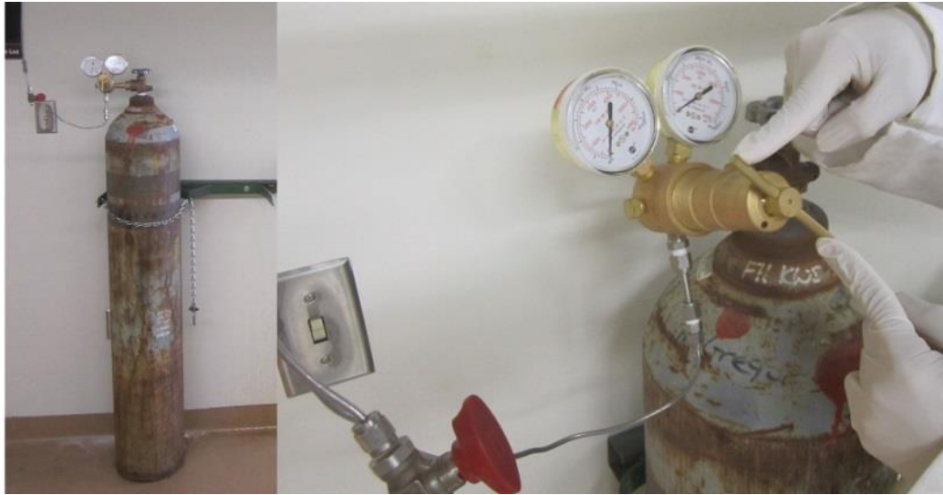
Figure 17: Nitrogen Tank, Pressure Regulator, and Bleed Valve
