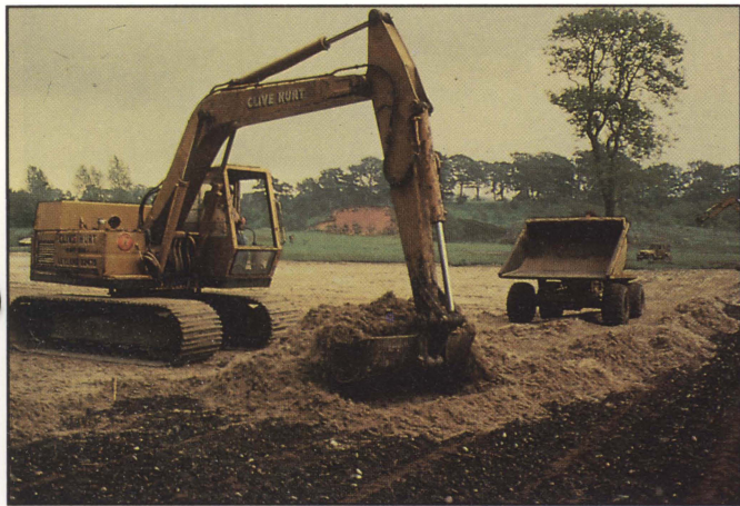
▲ Figure J-3. A back action bucket unit being utilized in rough grading the high-sand mesh matrix mix after dumping of the mix in piles on-site.
