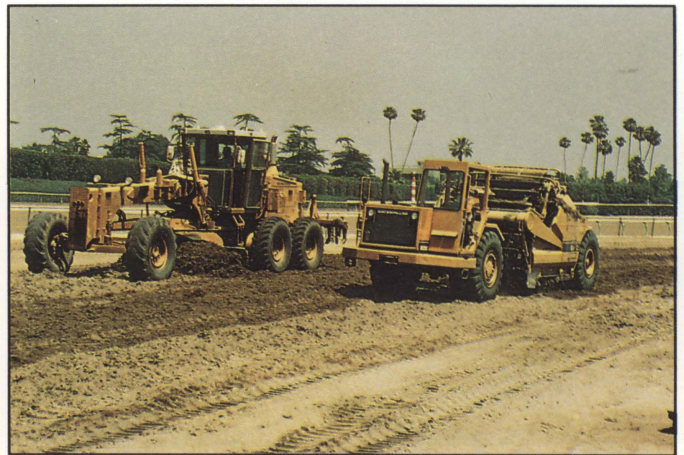
▲ Figure J-4. A road grader and elevating scraper grading and removing excess windrowed mix.
