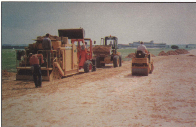
▲ Figure J-7. A machine for continuous installation of the mesh element-high sand matrix to a firm, controlled depth of 150 mm (6 in.).
