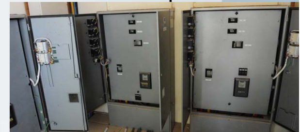
5 Power Panel Sub-meters
