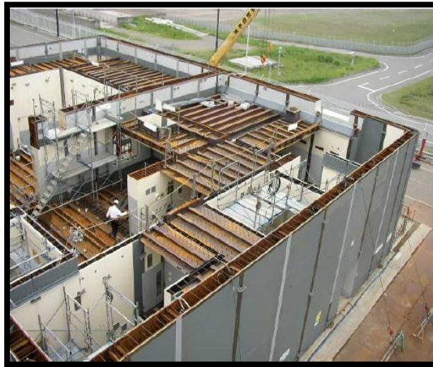
Figure 41 Steel-concrete composite concrete (IAEA, Advanced construction methods for new nuclear power plants, 2012)
