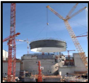
Figure 37 Assembling prefabricated parts (IAEA, Advanced construction methods for new nuclear power plants, 2012)
