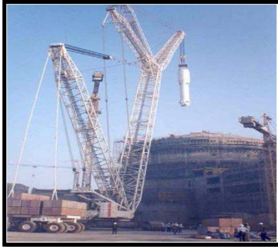
Figure 35 A steam generator installs with VHL crane (IAEA, Advanced construction methods for new nuclear power plants, 2012)
