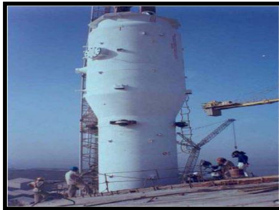
Figure 36 Open top installation for a steam generator (IAEA, Advanced construction methods for new nuclear power plants, 2012)
