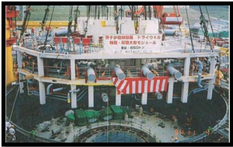
Figure 38 Installing the upper drywell super large scale module (IAEA, Advanced construction methods for new nuclear power plants, 2012)
