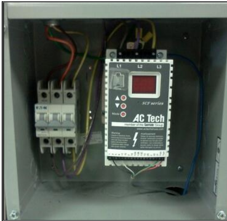
Figure 3-15: The SF430V mounted in an electrical enclosure box.
