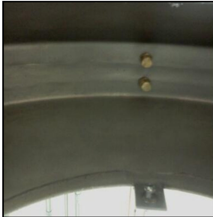
Figure 3-25: The argon spray nozzles mounted to the top of the catch pan.
