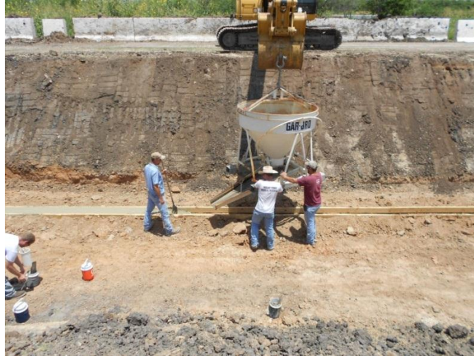
Figure D.3 Construction of the leveling pad where the first layer of panel will rest
