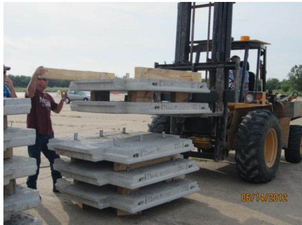
Figure D.1 Precast concrete panels of the TL-5 MSE wall test installation
