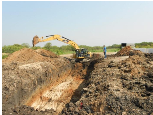
Figure D.2 Excavation for construction of the TL-5 MSE wall test installation
