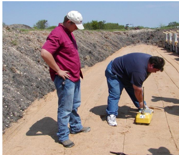
Figure D.7 Nuclear density test to determine the in-situ dry unit weight and water content
