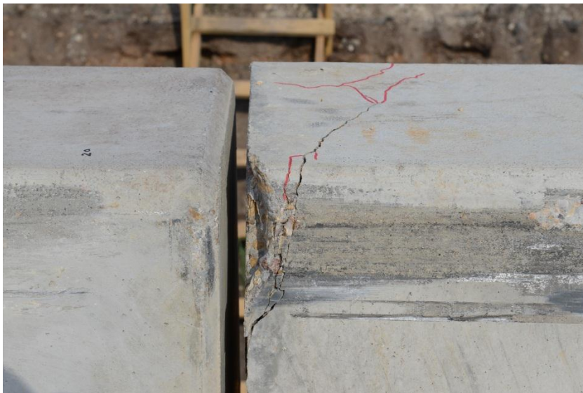
b) Crack at the barrier joint (B2-B3) due to the trailer impact
