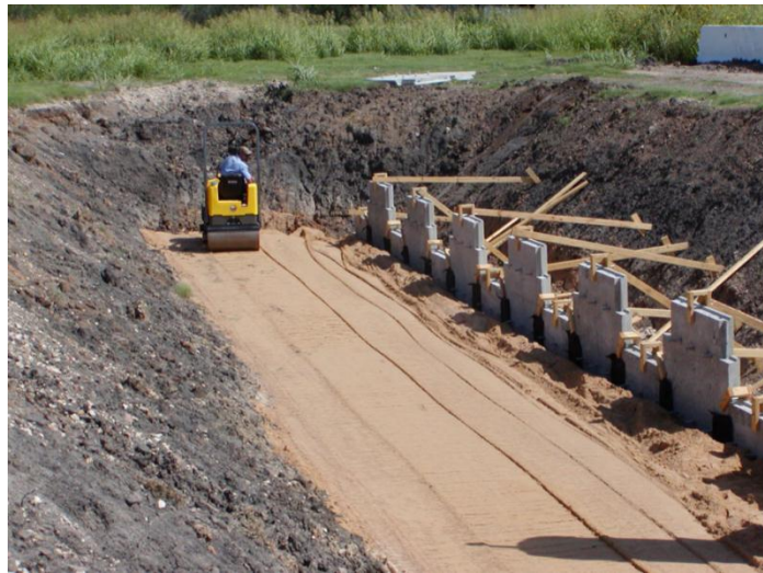
Figure D.5 Compaction of the backfill material below the bottom layer of strips
