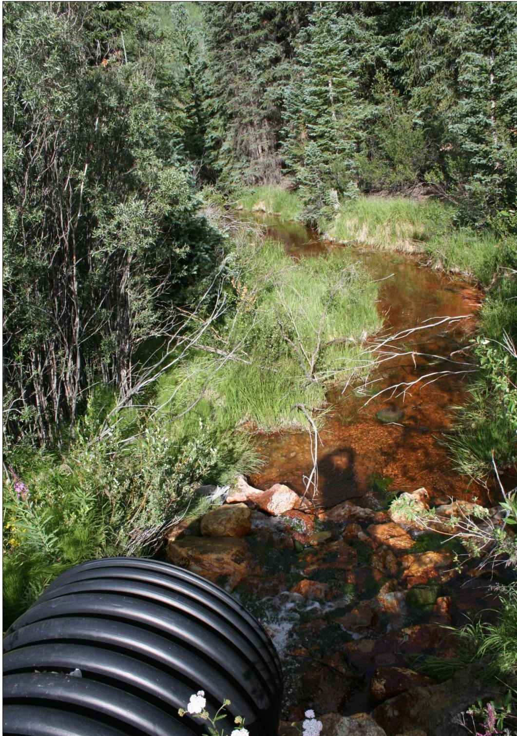
PHOTOGRAPH 28. Culvert under Highway 550 draining orange-colored water from the west side to the east side of the former glacial lake.
