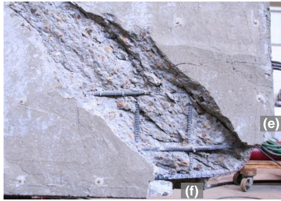
(b) After removal of Spalled Concrete at Outside Corner of Joint Region
