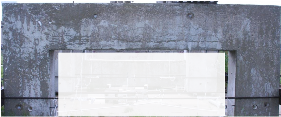
Figure 4-22 Crack Pattern of Specimen 3 after 748 Days of Exposure
