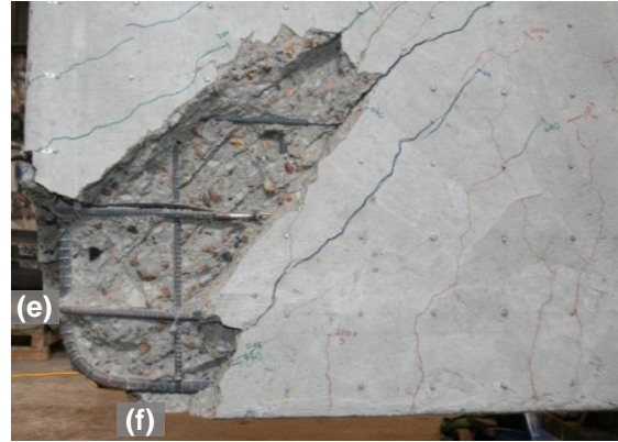
(b) After Removal of Spalled Concrete at Outside Corner of Joint Region
