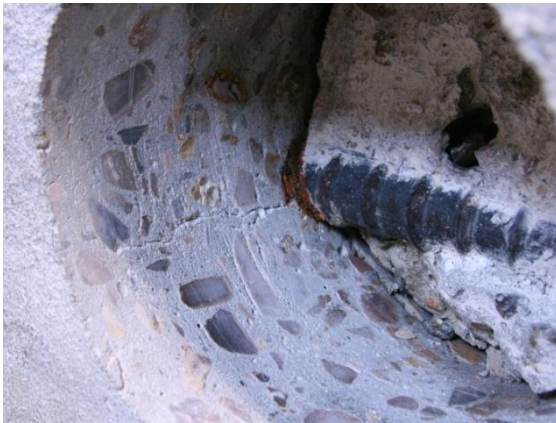
(c) Crack from surface to Reinforcing Steel (Core 2)
