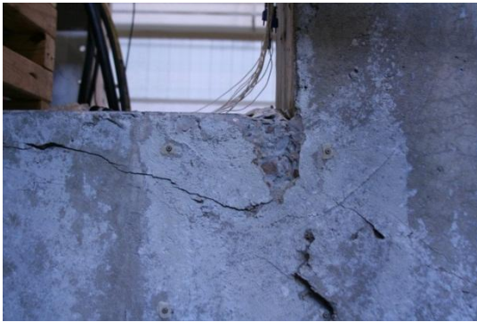
(c) Crushed Concrete at Inside Corner of Joint Region
