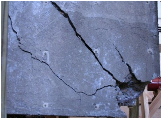
(a) Failure at Outside Corner of Joint Region
