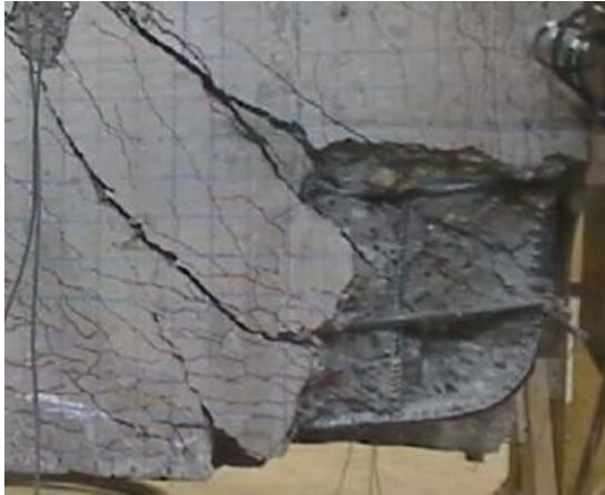
(a) Failure at Outside Corner of Joint Region
