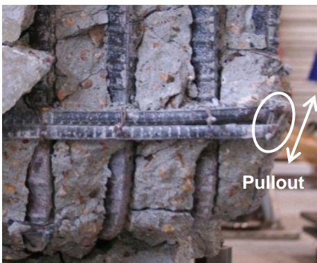
(e) Debonding of U-Shaped Steel Bars
