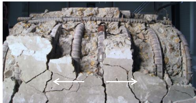
(f) Bulging of U-Shaped Steel Bars and Out-of-Plane Bending of Longitudinal Steel Bars
