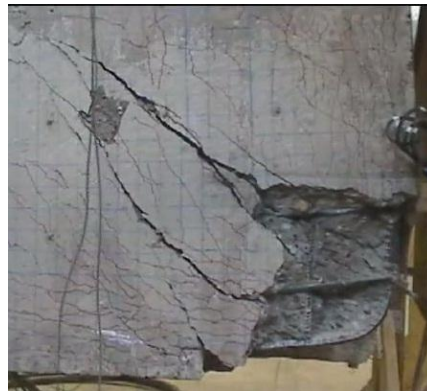
(c) Singly Reinforced Beam Region (after Failure)
