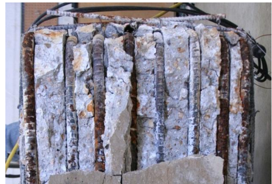
(f) Bulging of U-Shaped Steel Bars, Out-of-Plane Bending of Longitudinal Steel Bars, and Steel Corrosion
