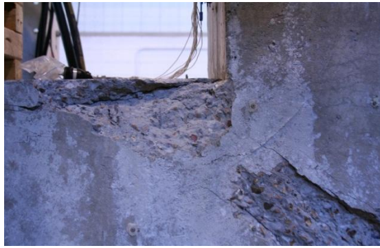
(d) After removal of Spalled Concrete at Inside Corner of Joint Region
