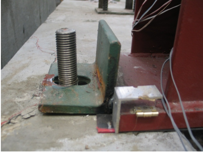
Figure 2-3. L-shaped angles welded to the short pedestal (S) base plate (anchor bolt nut not shown)
