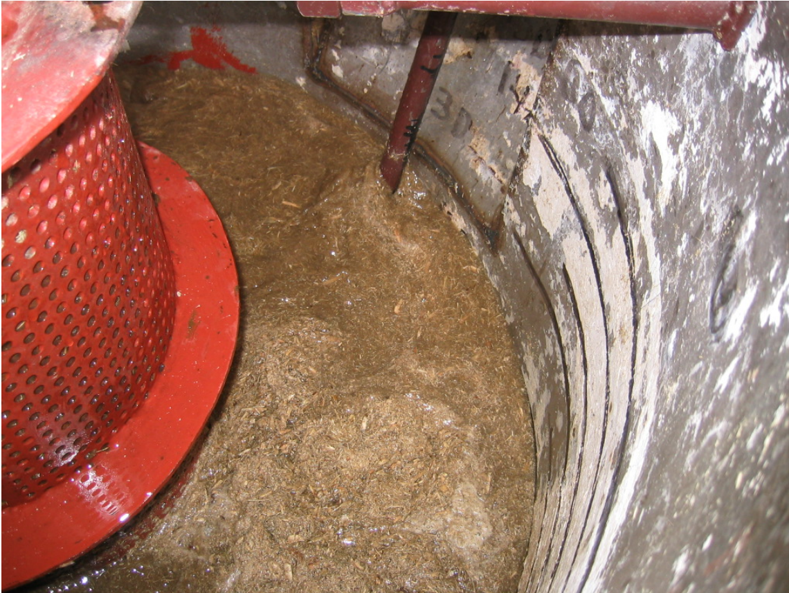
Figure 2.14 Photograph of inside the tank during operation.
