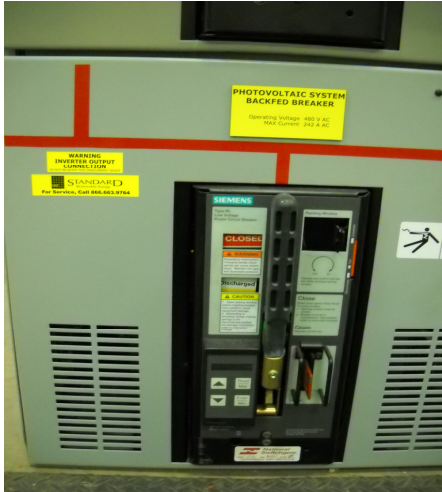
Figure 7. Inverter interconnect circuit breaker
