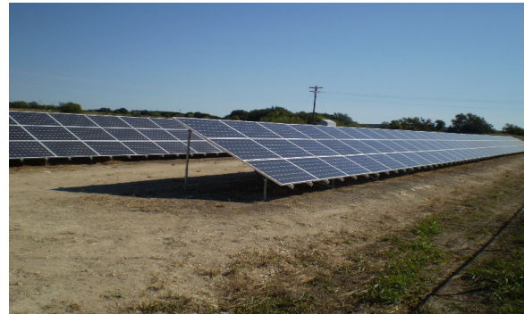
Figure 1. Commercial PV Installation
