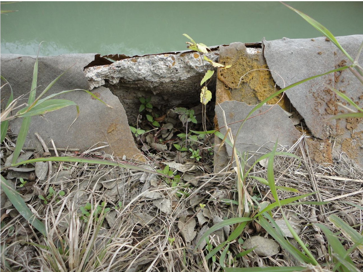
Figure 13. Damage caused by the sharp edge of the concrete underneath
