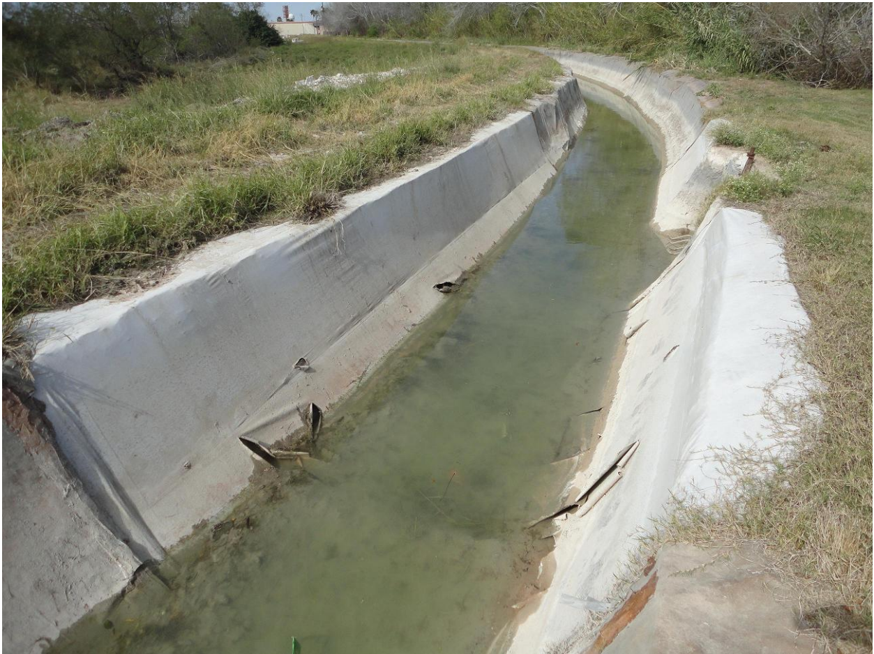
Figure 9. PVC Alloy liner damage.
