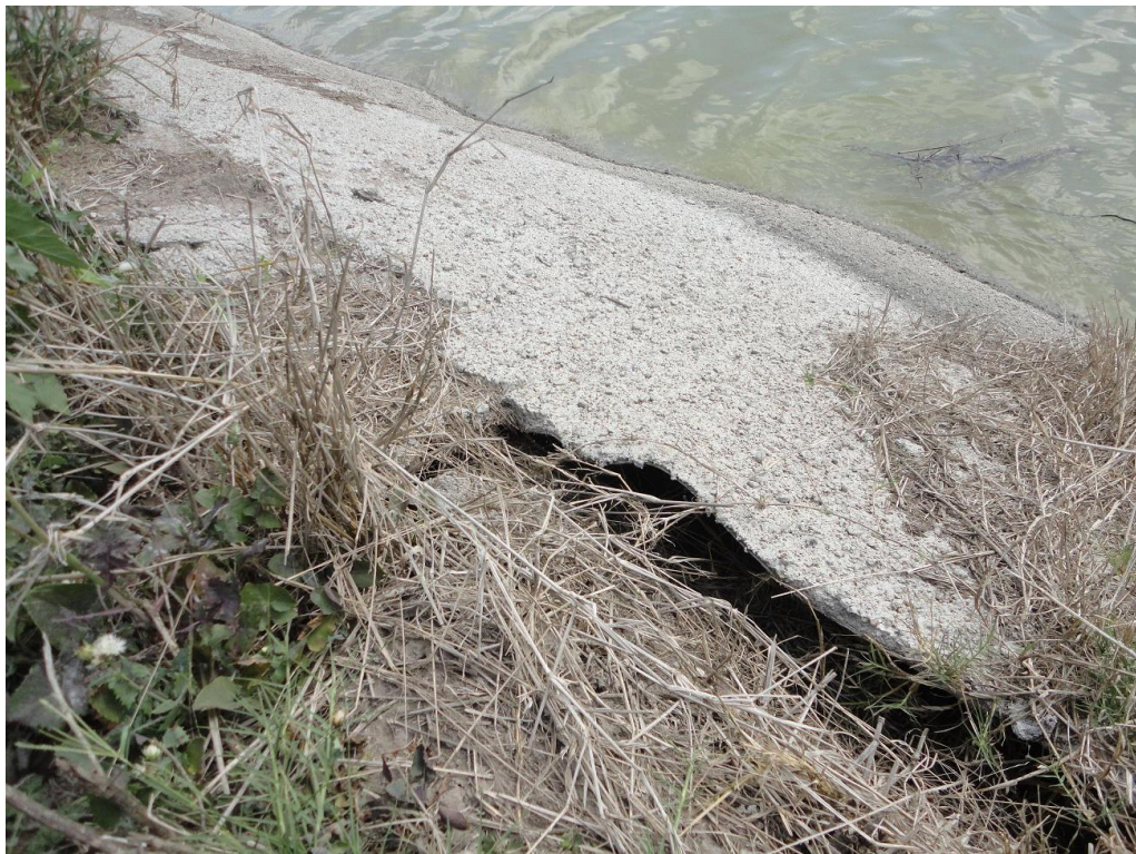
Figure 6. Erosion underneath the synthetic liner
