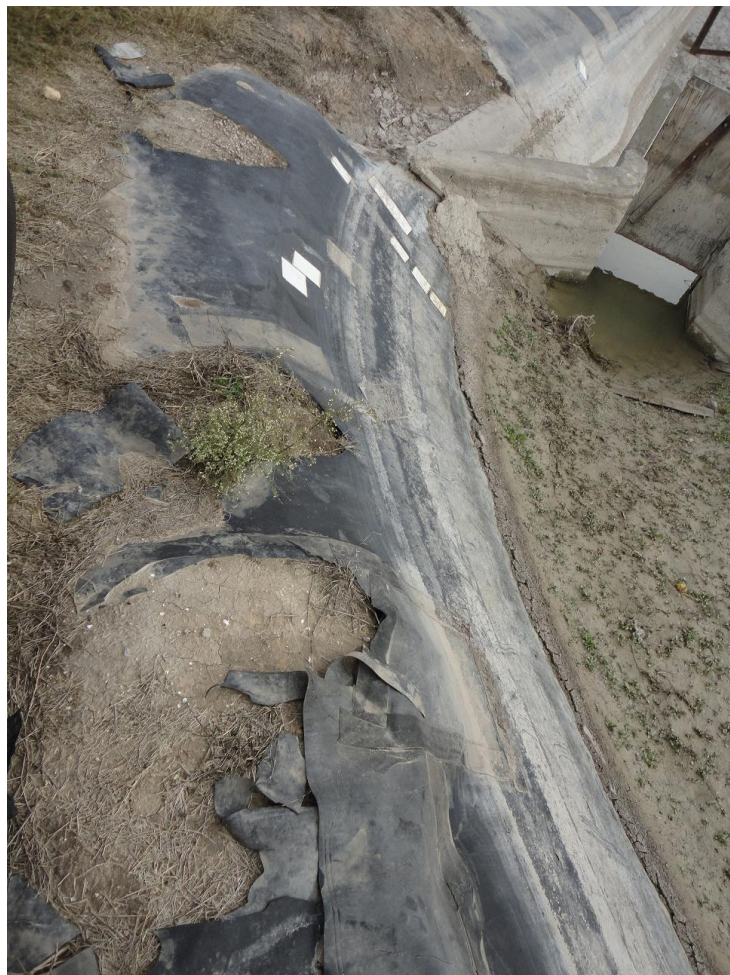
Figure 7. Damage on the anchor likely caused by mowers.
