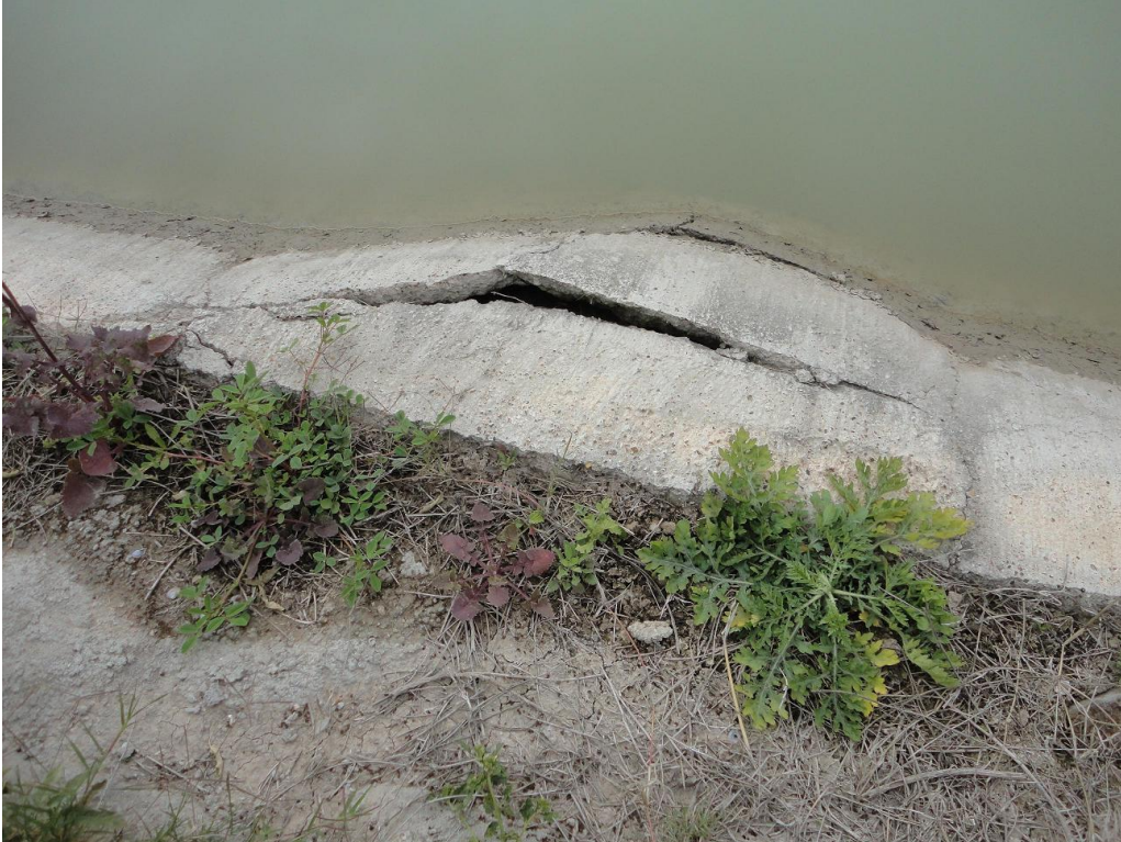
Figure 5. A buckle on the shotcrete protective barrier
