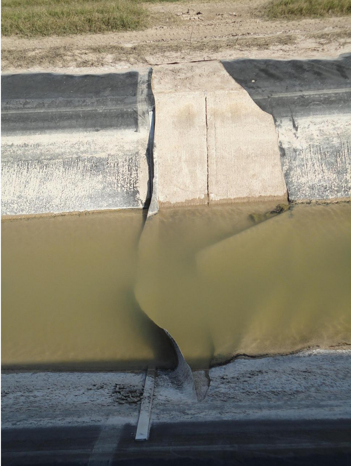
Figure 12. Steel anchors added to try to keep the liner from shrinking and floating
