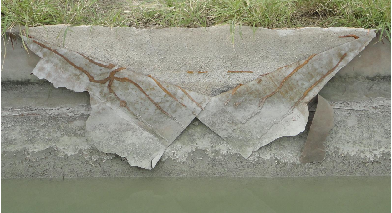
Figure 14. Polyurethane liner hanging off the canal side
