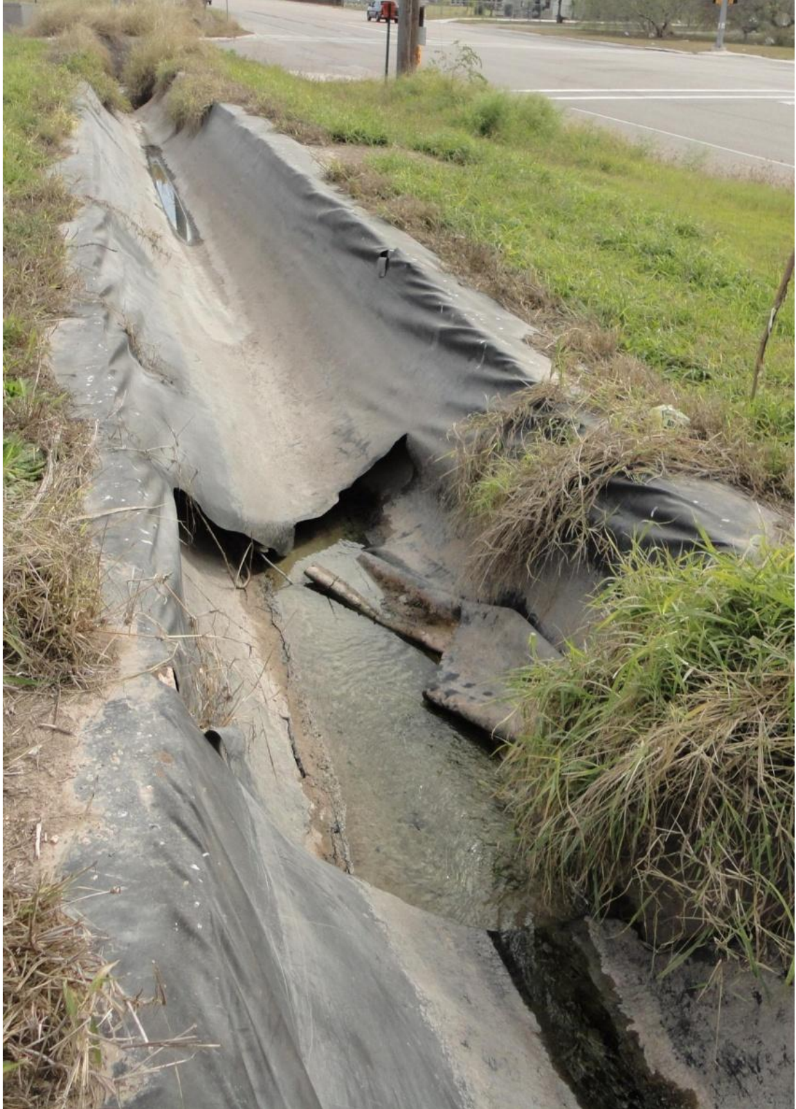
Figure 11. Cuts/tears caused by vandalism or traffic, and quickly enlarging due to shrinkage
