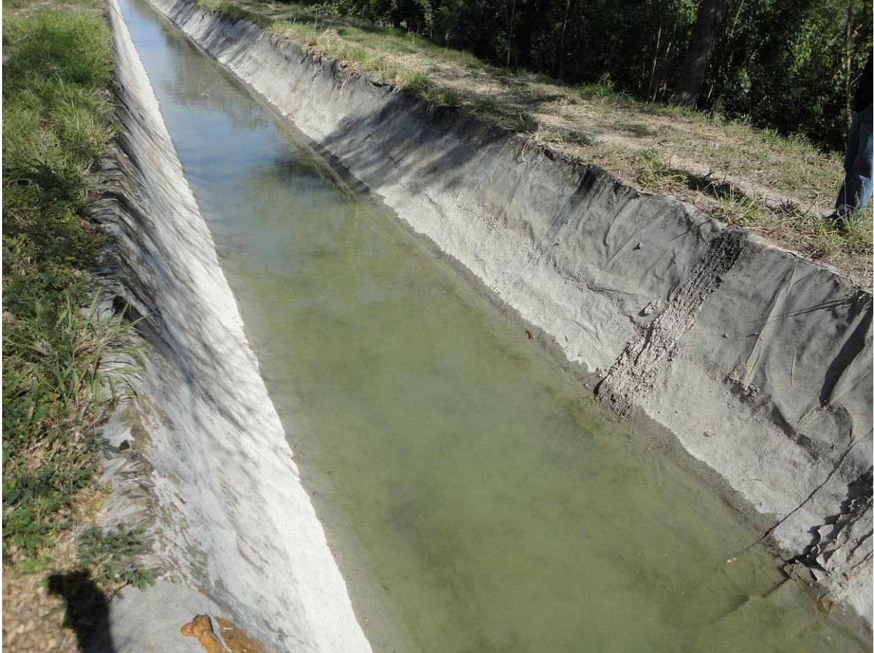
Figure 16. One polyurethane-lined segment in Fair condition after 12 years of use
