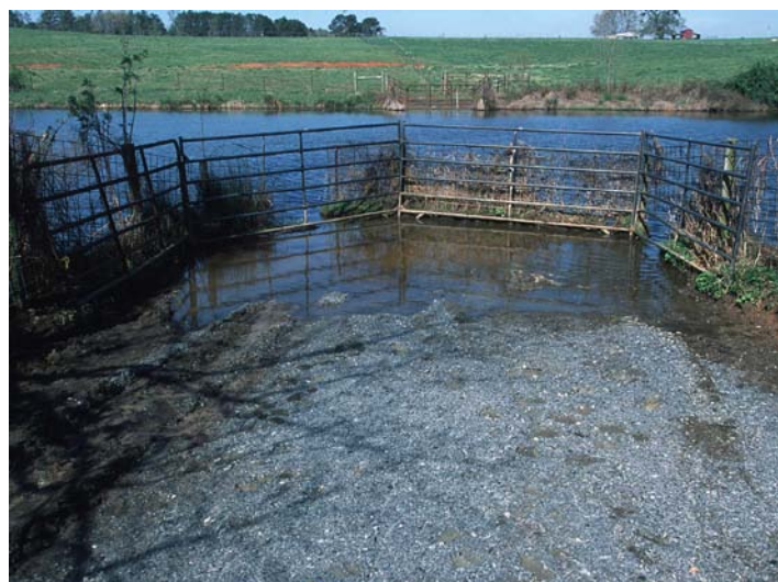
Figure 13. Example of an in-stream watering point installed to prevent cattle from disturbing the adjacent riparian area. Photo courtesy of Jeff Vanuga, USDA-NRCS.
