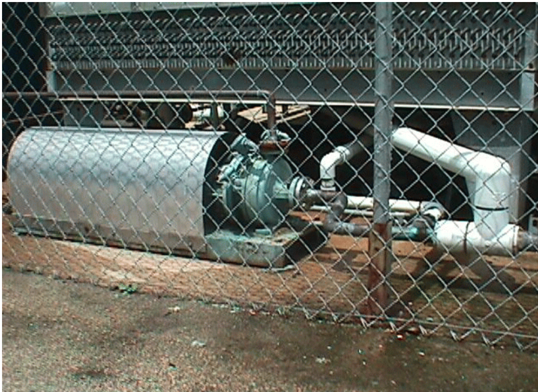
Fig 98. Re-circulation pump of the heat exchanger
