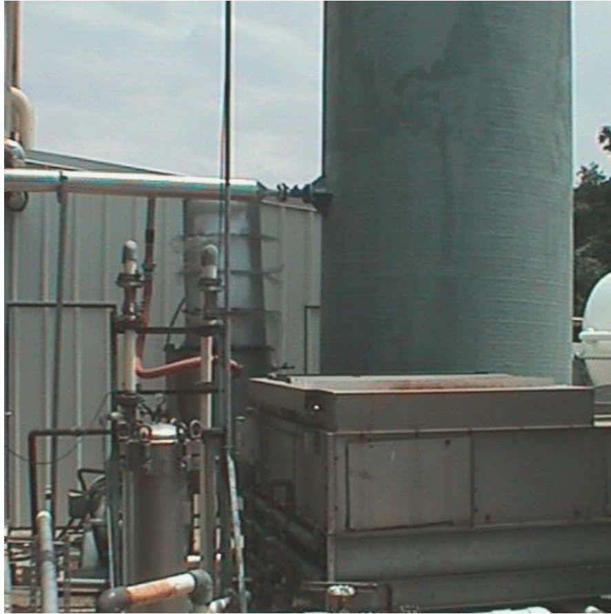
Fig 96. The main supply tank, heat exchanger and water filter
