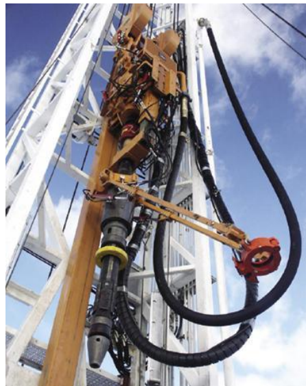
Fig. 19—Casing drilling equipment mounted on the rig: casing drive system + top-drive (Tesco 2008).
